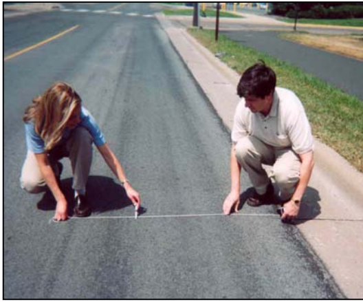
Jill Thomas, MAPA, and Dr. Mihai Marasteanu, University of Minnesota, check for distresses on the busway.
